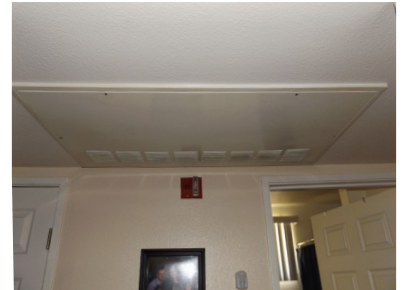
Fan Coil Location, Typical
