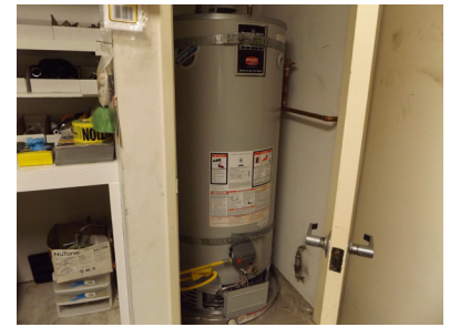
Gas-fired Water Heater
