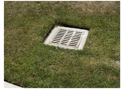
Typical Area Drain
