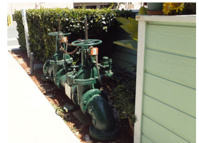
Backflow Device Location
