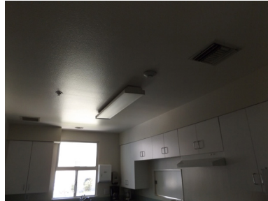
Typical Fluorescent Fixture
