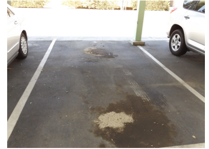
Degraded Surface Condition
