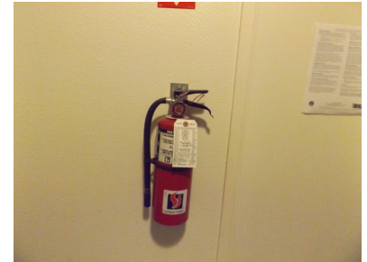
Typical Extinguisher Location
