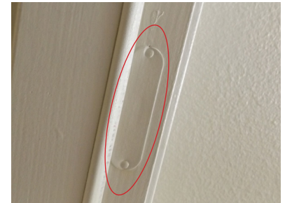
Painted-over Fire Rating Plate
