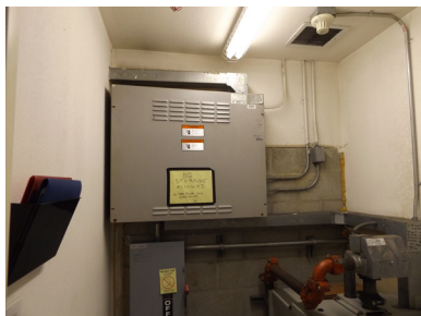
Elevator Equipment Room, Angle 1
