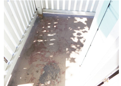
Stained Traffic Coating
