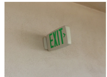
Exit Sign, Typical
