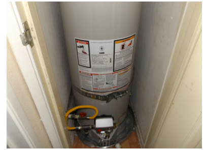
Typical Unit Water Heater
