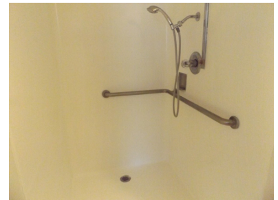
Typical Unit Shower
