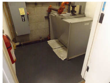
Elevator Equipment Room, Angle 2
