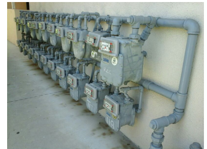
Unit Building Gas Meter, Typical
