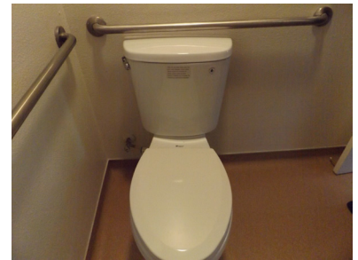
Typical Unit Toilet
