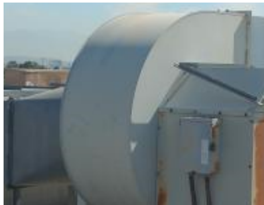
Building A Roof Fan
