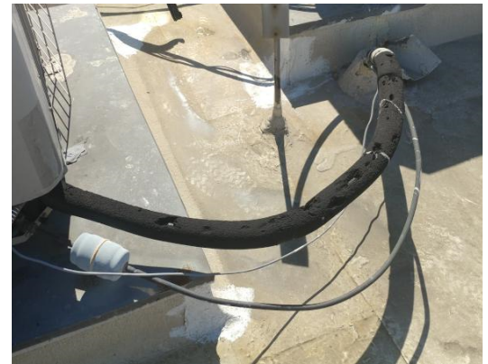
Community Room Air Handler
