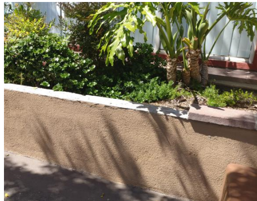
Missing Cap Section at Community Room
