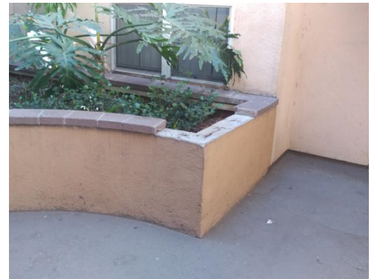
Missing Cap Section
