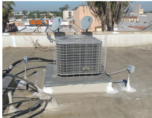
Roof Mounted Condenser
